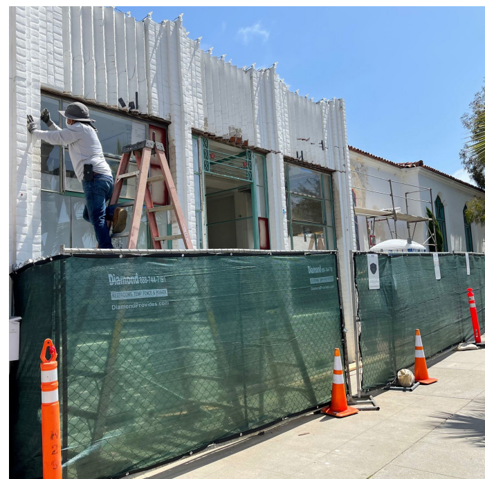
Renovation of the historic Parker Building and the façade of the Girard Avenue side of the William Templeton Johnson Building has already begun.
